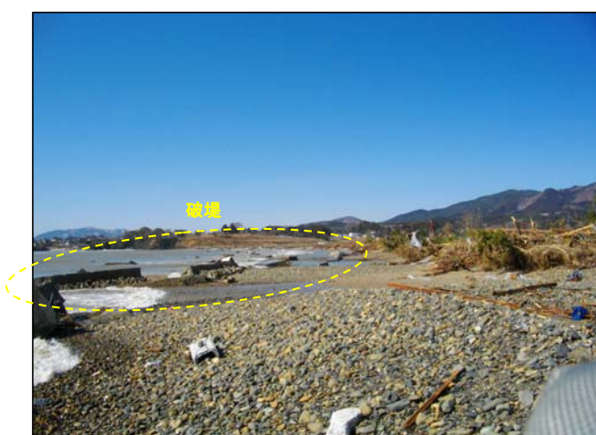
④堤防破堤
