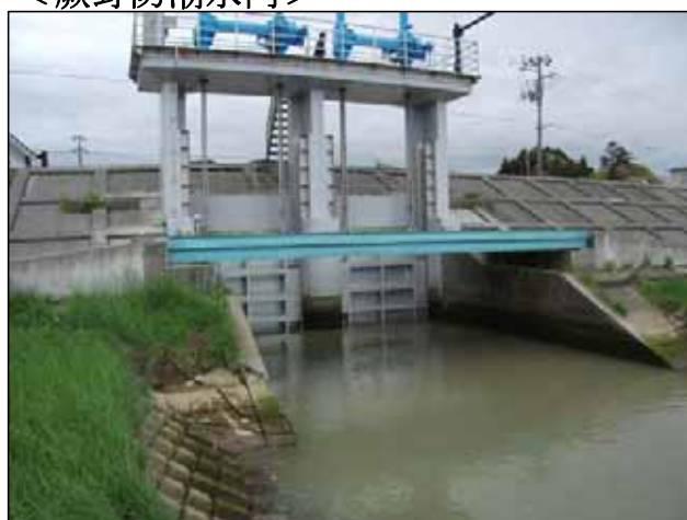
①蕨野防潮水門被災前
