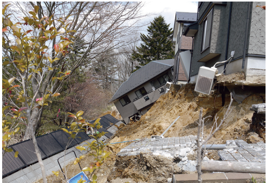
Damage to hillside residential land in Seikaen, Aoba Ward, Sendai City (Photo: Sendai City)
