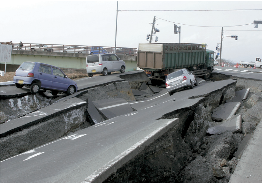
March 11: Road damage near Eai Bridge in Furukawa, Osaki City (Photo: Osaki City)
