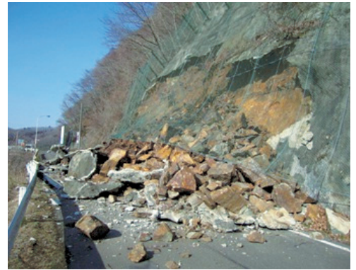
Damage to road embankments in the Hasekura area of Kawasaki Town (Photo: Kawasaki Town)
